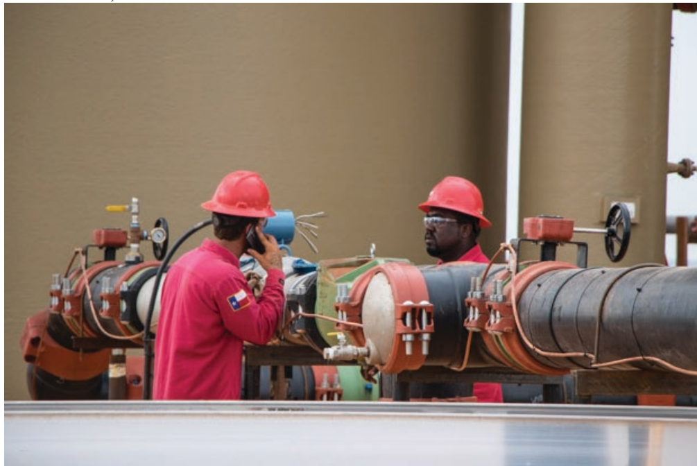
Electricians perform final checks on equipment nearing a tank battery at the Barton facility.
