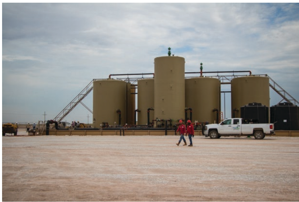
Electricians complete last-minute work at Newfield's Barton Water Recycling Facility near Calumet, Okla.
